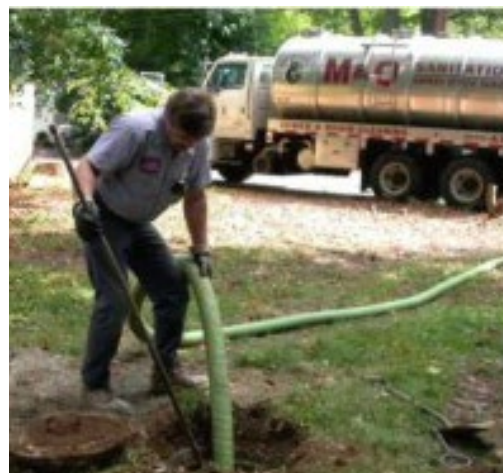
Figure 3.6.1. Pumping the septic system. Credit: Conasauga River Alliance ( www.conasaugariver.org ).
