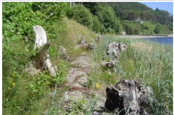
Figure 1.3.2. Bulkhead removal - before, during and after. Credit: King County Water and Land Resource Division.
