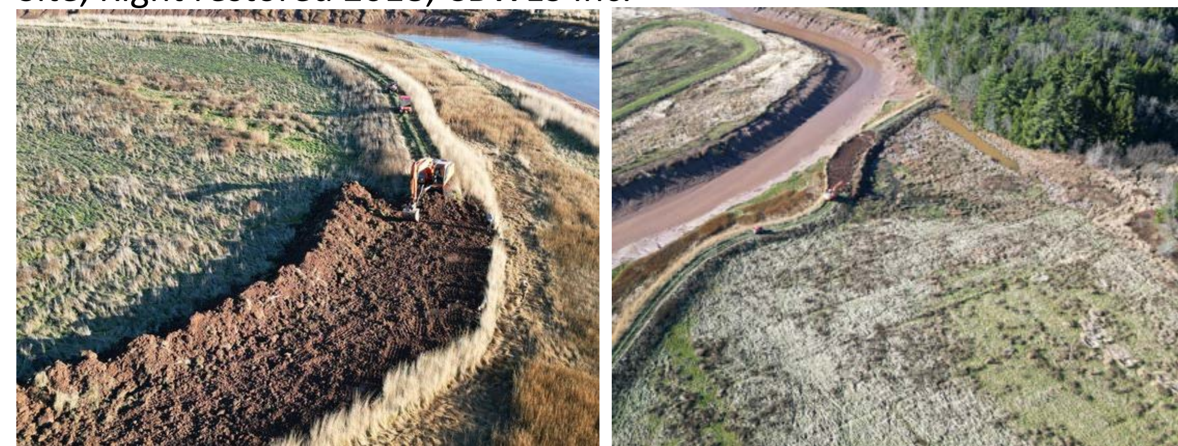
Earthworks at the Ksu'ksw Mqoqt/Hemlock Marsh Managed Realignment Site, restored 2022, CBWES Inc.
